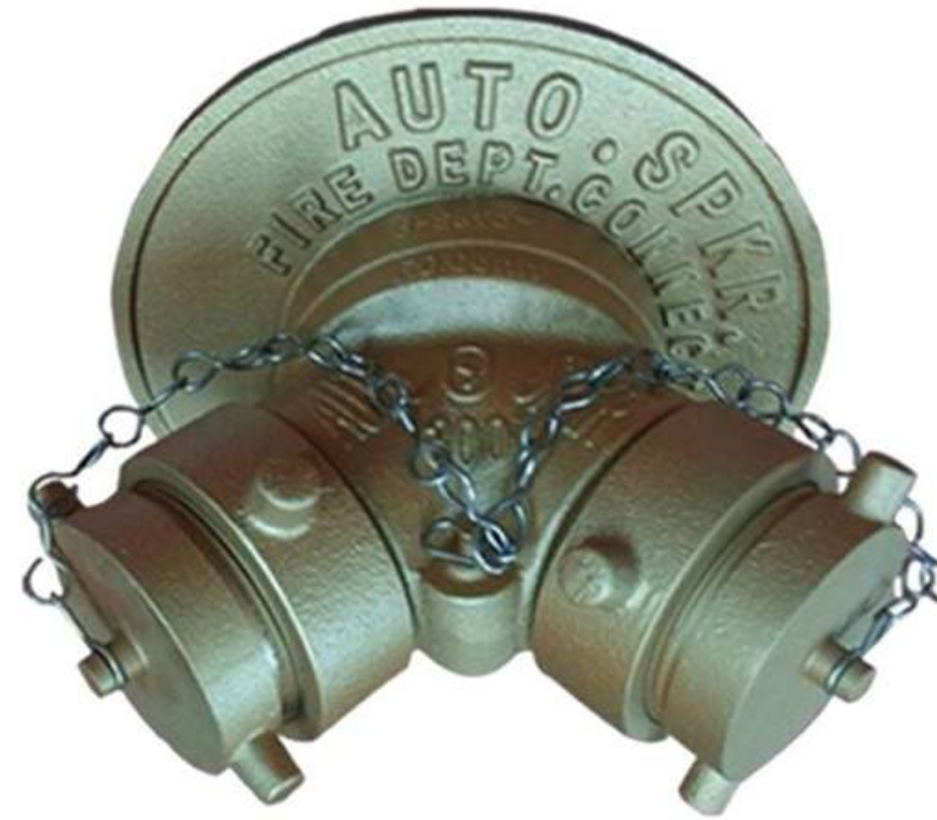
FIRE DEPARTMENT CONNECTION
